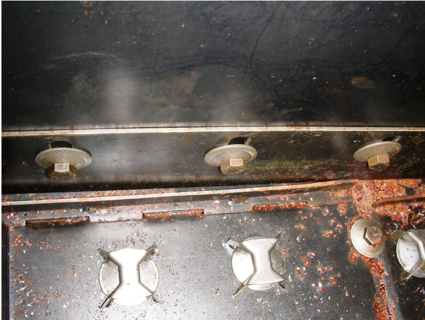
Incorrect Inlet Weir Clearance
