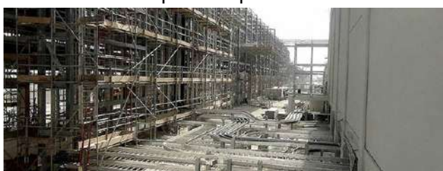
Figure 3 – Sadara Power and Piperack Interface (3)
