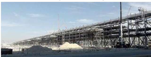
Figure 4 – Sadara 2km Interconnecting Facilities Piperack (3)
